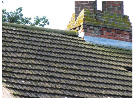
Photo 10: Gaps under lead flashing and missing mortar in ridge tiles
